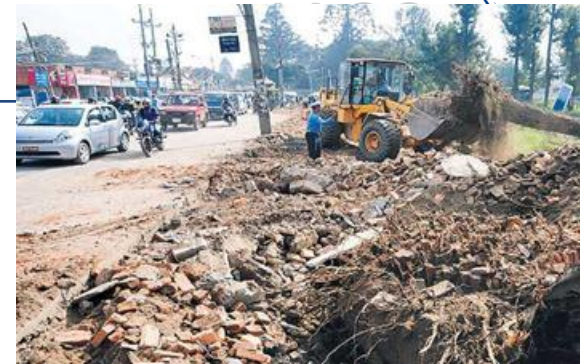
Poorly maintained roads
