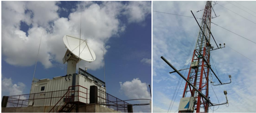
C Band Radar and instrumented Tower at NBNSCOE, Solapur
